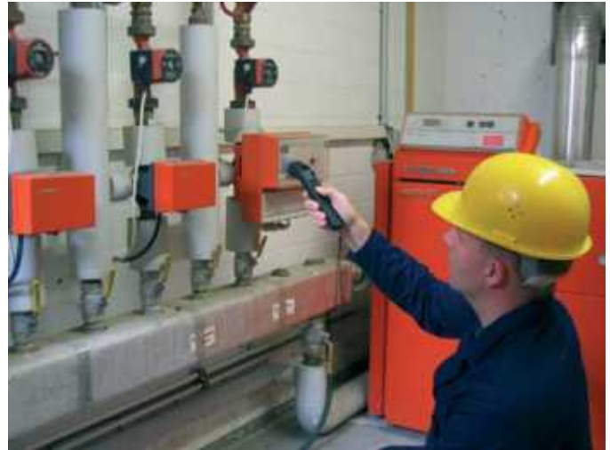
Checking the temperature of heating circles
