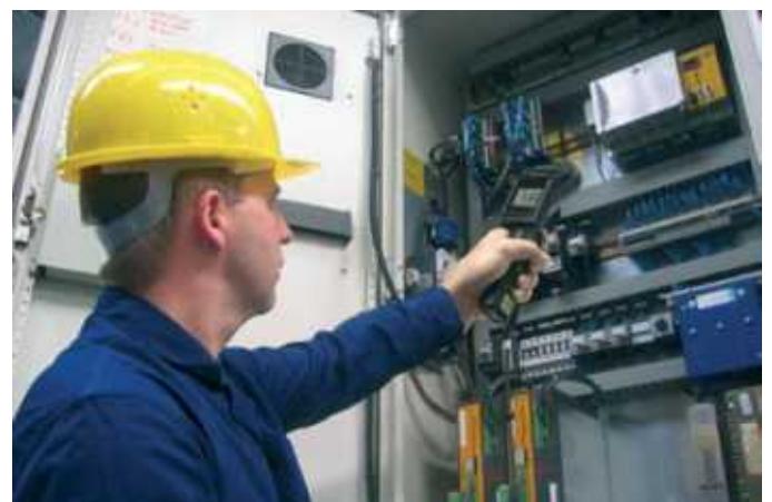
Detailed infrared temperature measurement of an electric control with the help of the installed close focus optics for 1 mm ranges of the optris LS LT
